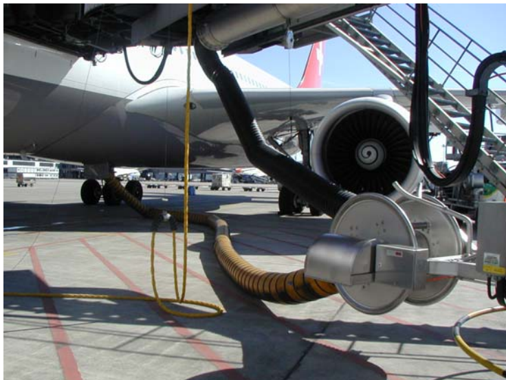
Figure 5-1: Fixed ground power systems
